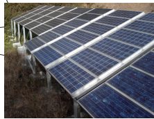
FIG. 18: SOLAR POWER CELLS
